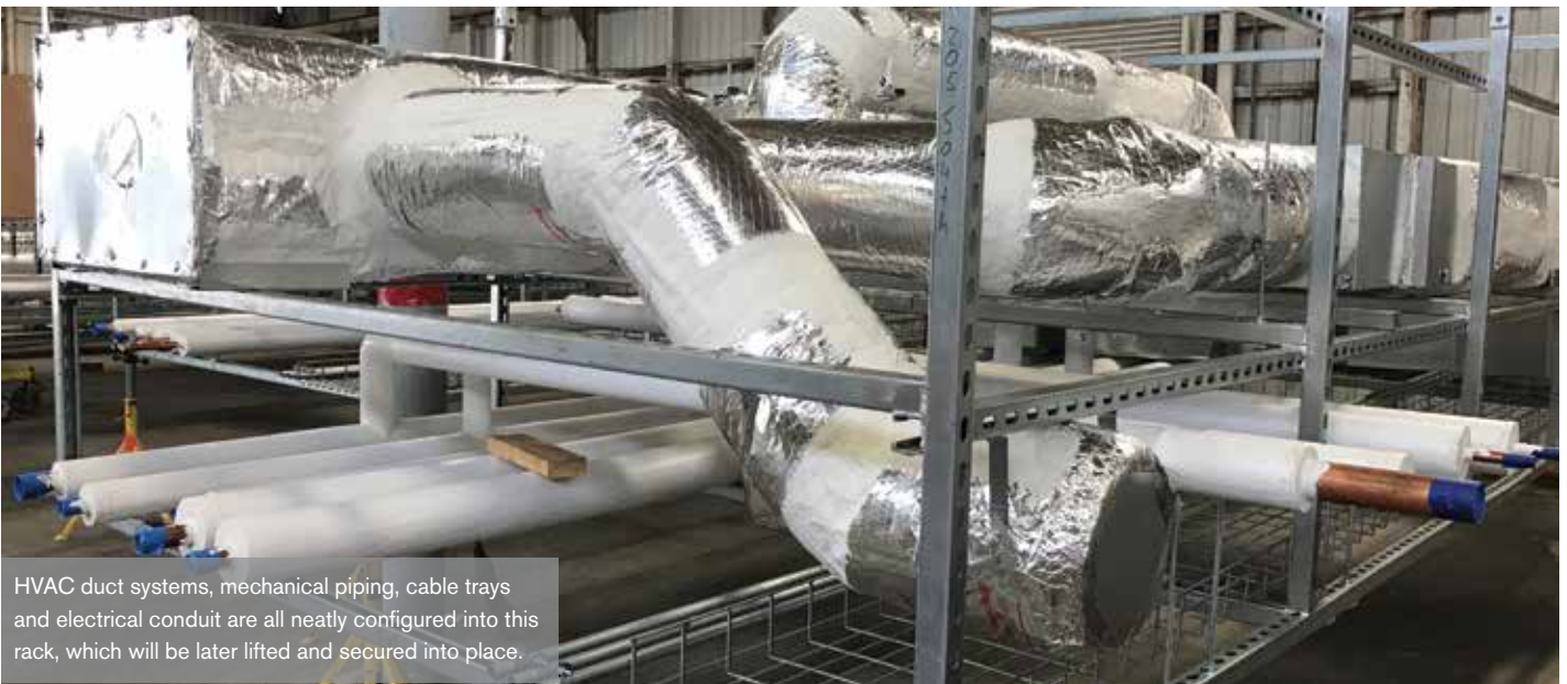
Mechanical piping is assembled, tested and insulated in a controlled warehouse environment, previous to installation the hospital.
